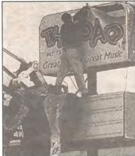
Chris Bellamy of Chuck's Construction rode the excavator bucket up to retrieve the sign as a souvenir for the Worleys, owners of the property. The Pad, a landmark in Myrtle Beach, is being torn down to make way for a parking lot.
